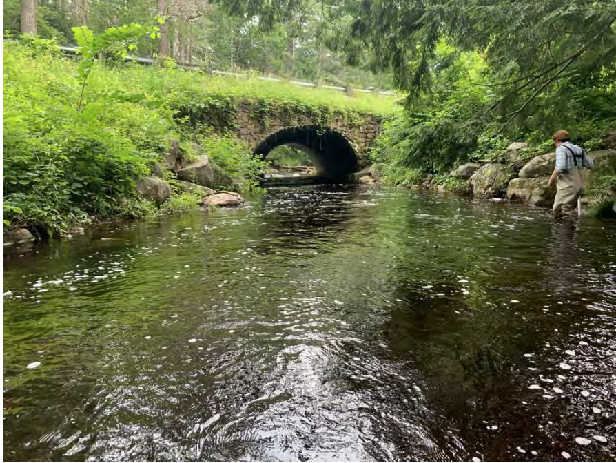
Photo 7. The inlet and out of the High Street culvert crossing are armored with riprap.
