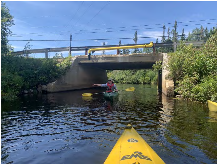
Photo 26. Reach 3 flows through a box culvert under New Road at approximately its midpoint, revealing deteriorating headwalls and wingwalls, and erosion around the structure.
