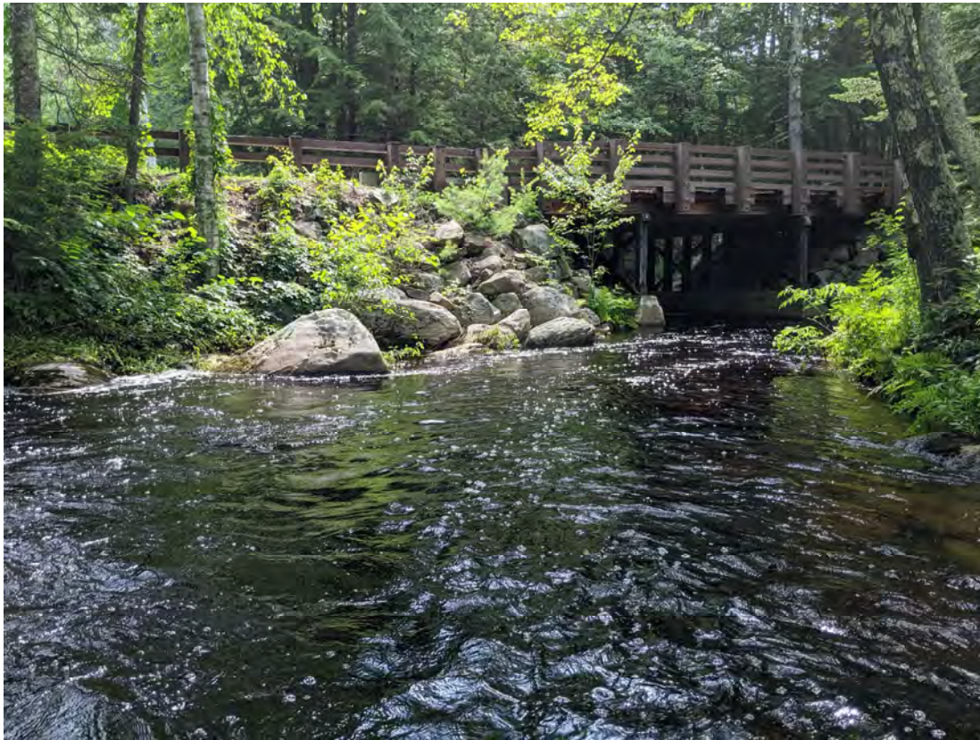
Photograph 23: County Road crossing of Melvin River, note poor alignment with river
