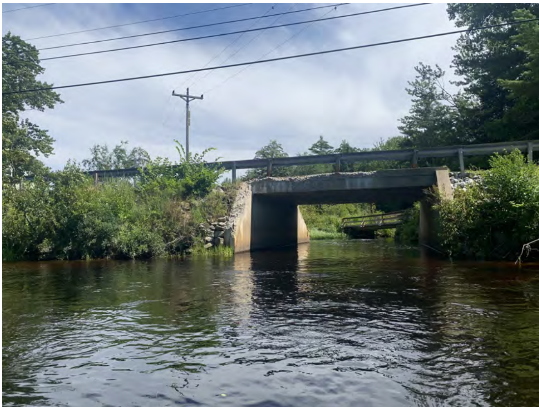
Photograph 20: New Road crossing of Melvin River, note erosion on left side (right bank)
