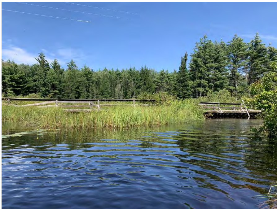
Photo 24. The Snowmobile Trail #1 crossing was nearly submerged due to woody material caught on and blocking flow through the structure in addition to backwatering effects from a large beaver dam downstream.
