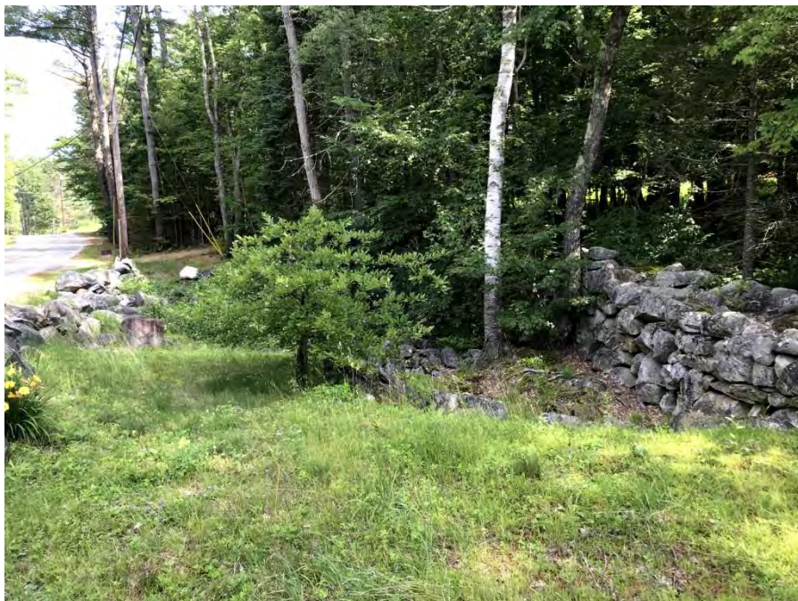
Photo 42. Remnants of dam structures, identified as Dam #2 Ruins, were found adjacent to (upstream and downstream) Reach 5.
