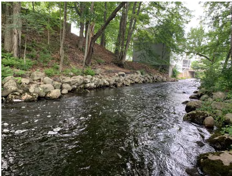
Photo 4. Dry-stacked boulder and concrete retaining walls line the banks of the lower segment of Reach 1.
