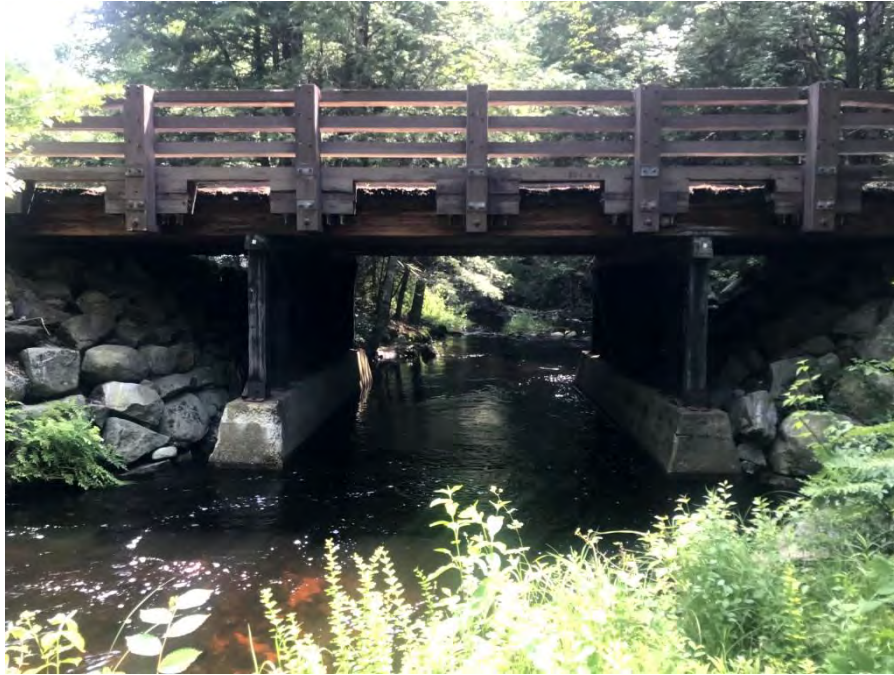
Photo 13. The County Road Crossing is an undersized open-bottom bridge with poor stream alignment.
