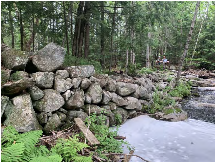
Photo 10. The Dam #1 Ruins were comprised of large and medium boulders stacked perpendicular across the river.
