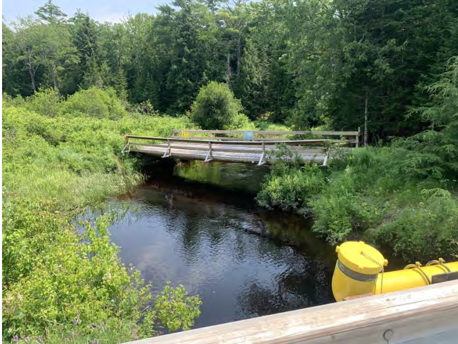
Photo 27. Immediately upstream of the New Road crossing is another Snowmobile Trail crossing (#2) spanning across Reach 3.
